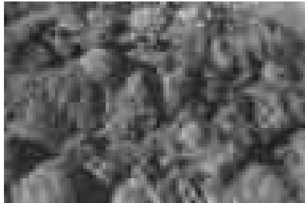
Fig.6.4 : Exfoliation (Flaking) and granular disintegration
