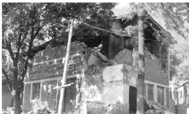
Figure 7.1 : A Damaged Building Due to an Earthquake
